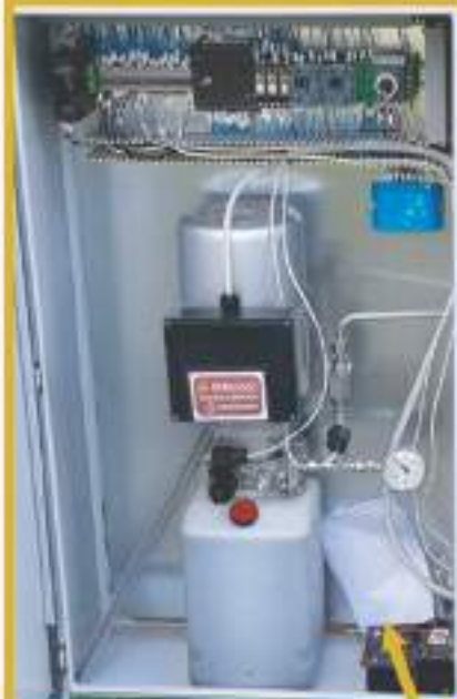
CENTRALINA E PLC
